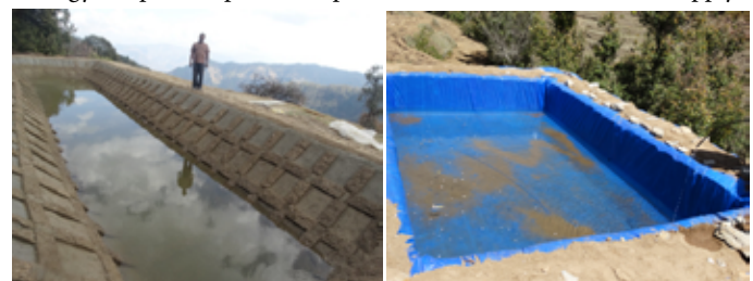
Fig. 4. Polylined tank with locally made bricks pitching Repaired cement tank with silpaulin
